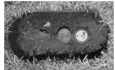
▲ outdoor water shut-off valve
