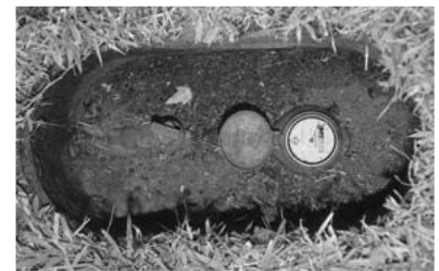
▲ outdoor water shut-off valve
