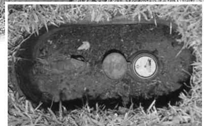
▲ outdoor water shut-off valve
